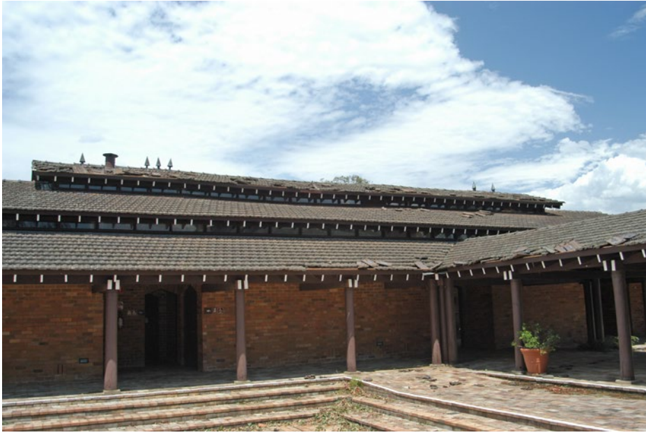
Storm damage to the campus and landscape on 4 December 2002
